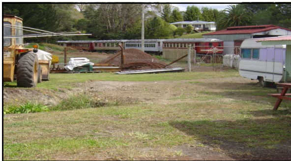
3/4 of the open drain is now covered and reclaimed as part of the accommodation area
